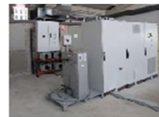
Li-ion battery, 50 kW, ½ hour
