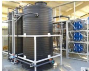
Flow battery, 50 kW, 4 hours
