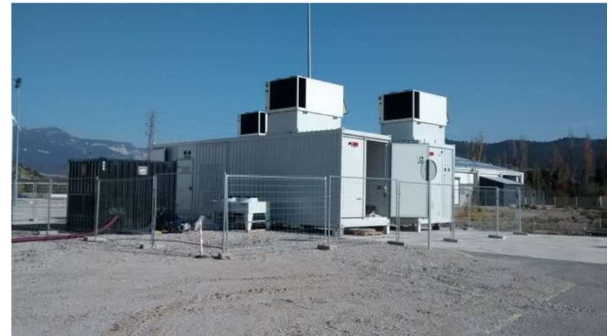
Ion Lithium Battery 1 MW, 500 kWh.
