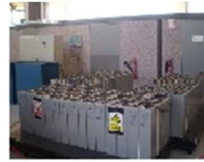
VRLA batteries, 50 kW, 2 hours
